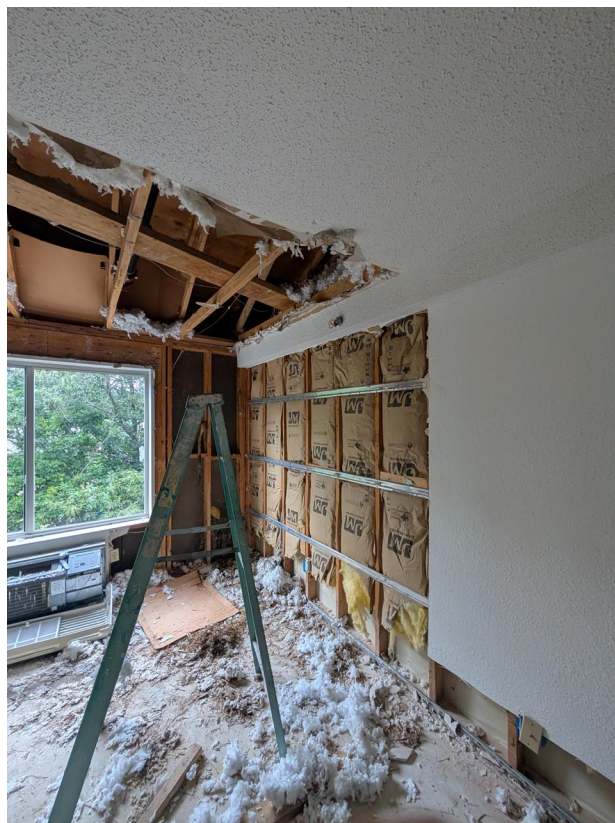
Exposed structure in room 325 and damaged areas
