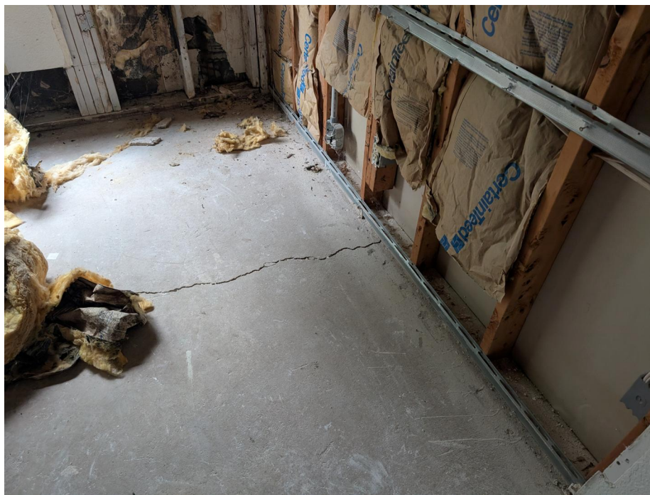
Crack in the slab of room 125 due to settlement
