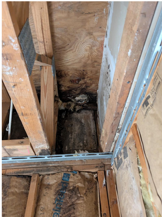
Water damage in the structure in room 225
