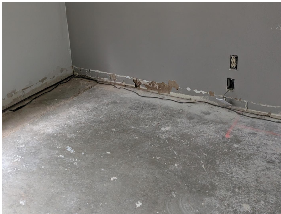
Gap between the drywall and slab due to settlement
