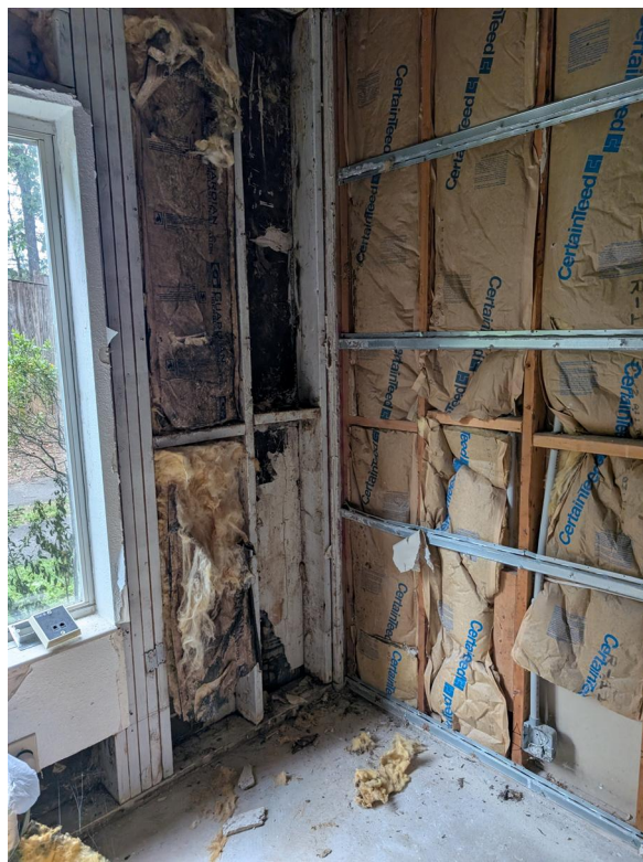
Exposed structure in room 125 and damaged areas
