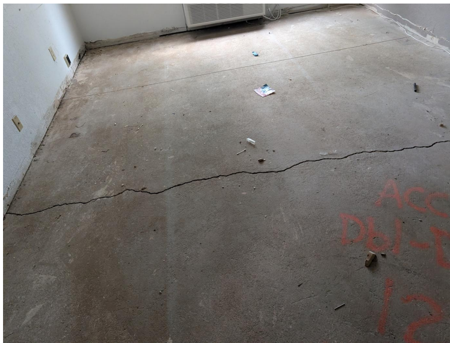
Crack in the slab on grade in the first floor due to settlement
