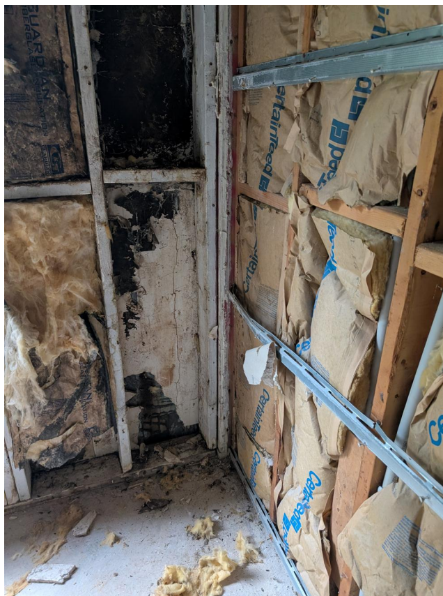
Water damage to the structure in room 125
