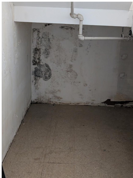
Water damaged area in the first level which is not exposed
