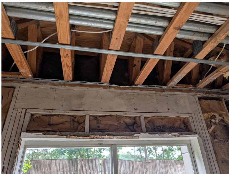
Exposed structure in room 125 and damaged areas
